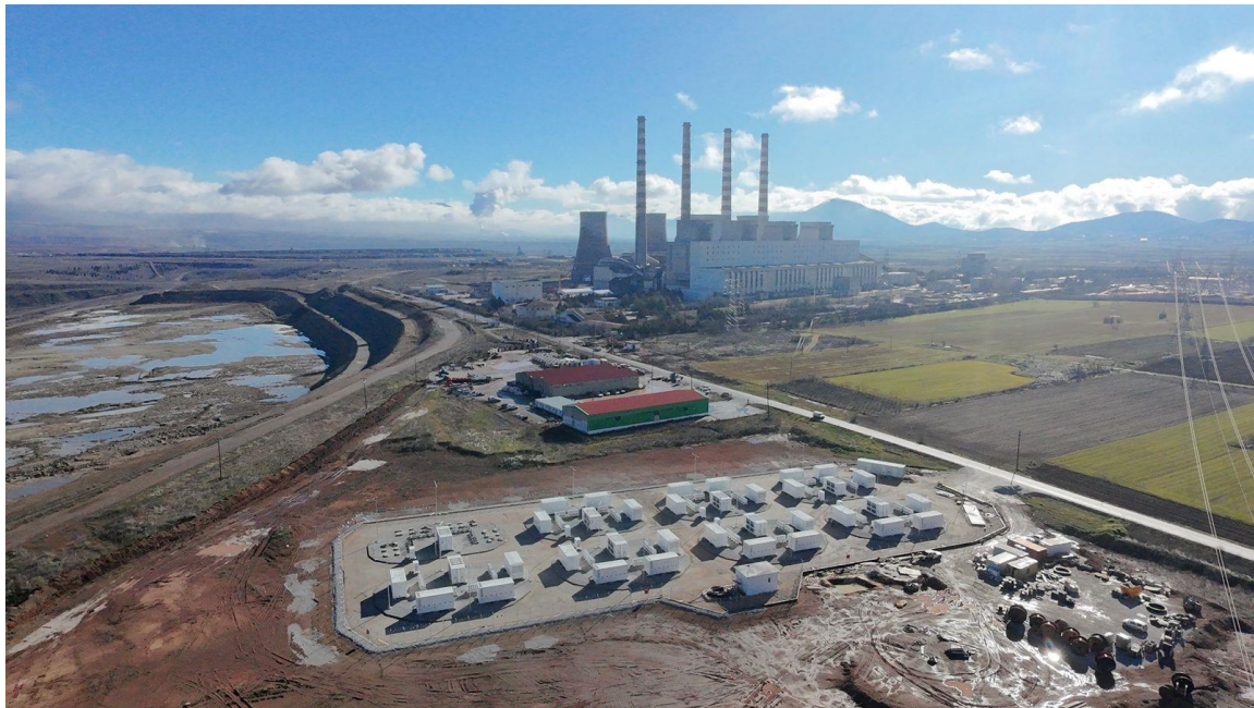
Figure 4: Battery array of the Ptolemaida IV Electrochemical Energy Storage Station. The Kardia Power Plant can be seen in the background, along with the location of the lower reservoir of the future pumped storage station.
